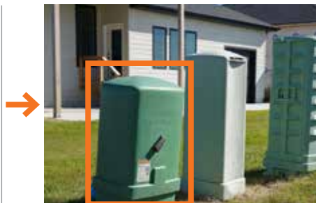
LES pedestal with proper clearance.
