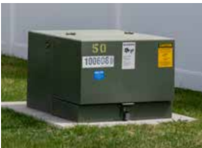
LES pad-mounted transformer with proper clearance.
