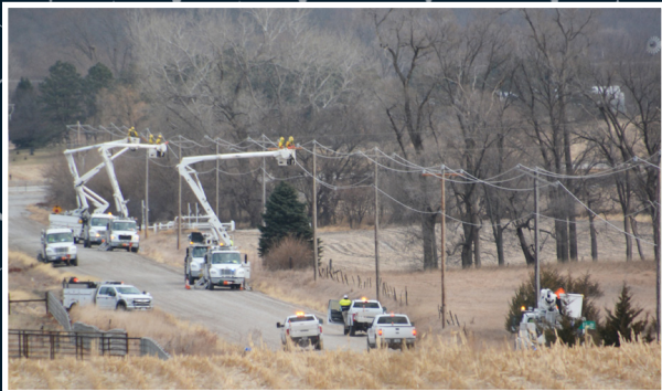
Crews repair powerlines and restore power after cold weather and high winds created galloping powerlines.
